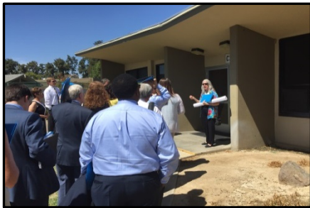
Former BHRS Director Dr. Madelyn Schlaepfer shows the CSU under construction to members of the MHSAOAC during their visit to Modesto on August 27, 2015.
